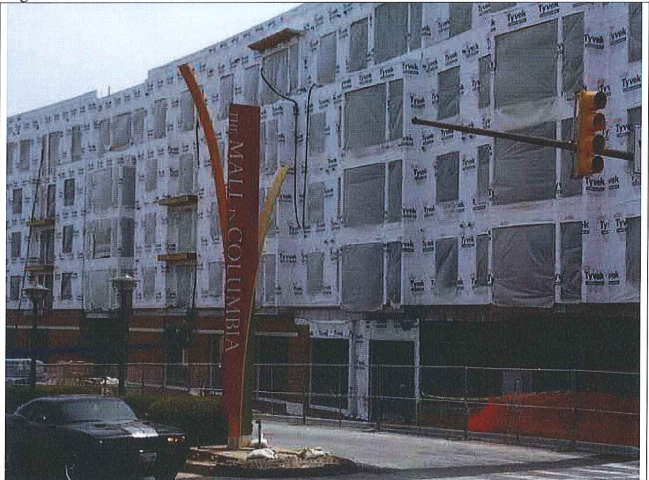
Construction of “The Metropolitan” seen from this vehicular entrance to the mall helps to illustrate the changes coming to Downtown Columbia
